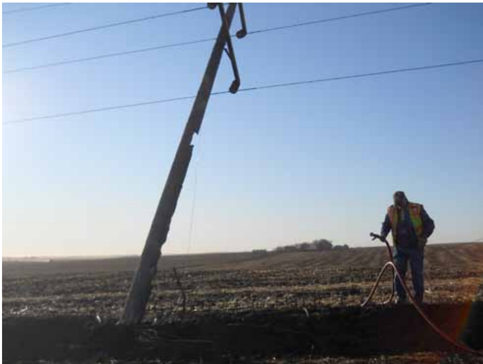
This transmission pole, above, leans severely after it was damaged by a fence line fire near Newkirk. In the photo at right, a pole near Modale was burned in a field crop residue fire. Both poles had to be replaced at the cost of several thousand dollars.
