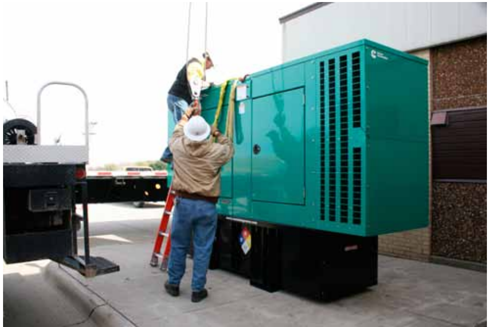
Dave Rolfes, procurement and equipment manager, on ladder, and Steve Haringa, crew foreman, unstrap the new standby generator after setting it in place with a boom truck.
