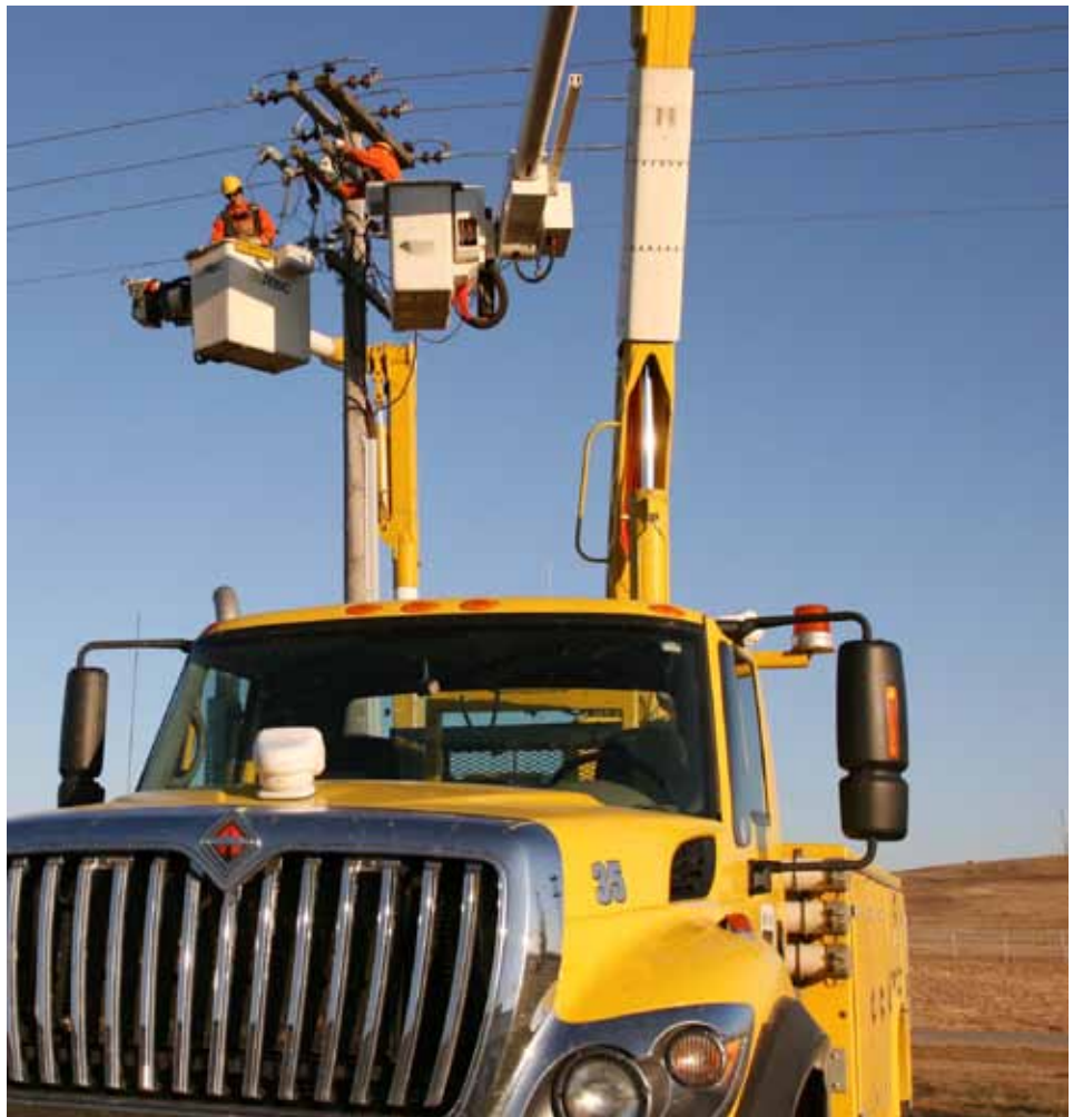
Crews from North West REC, which serves power to the NIPCO headquarters building, put up a new primary riser to feed NIPCO's new building transformer.
