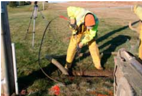
A contractor begins boring a route for the new underground electric service to NIPCO's headquarters building.
