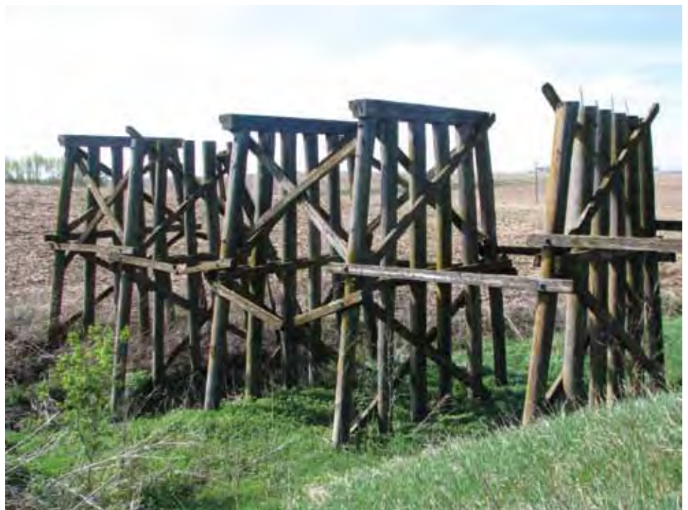
This is one of three abandoned railroad structures noted in the archaeological study required to apply for Federal Emergency Management Agency funding to retrofit 151.14 miles of NIPCO's oldest transmission line.
