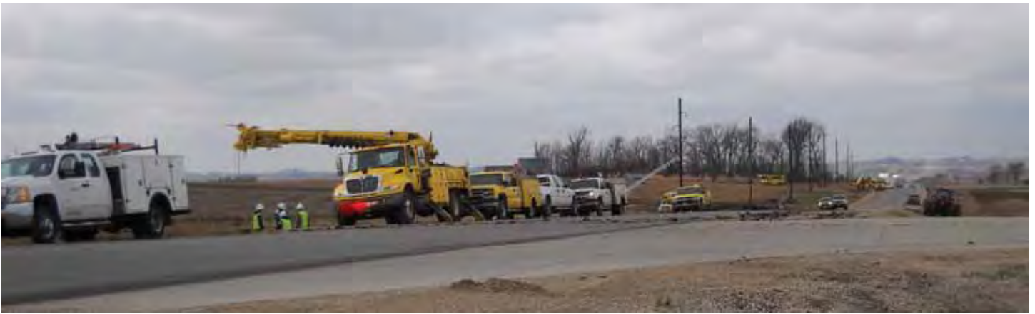
Crews from both NIPCO and North West REC worked together to replace eight downed poles and conductor on the tap line feeding the Galva Substation following the tornado.
