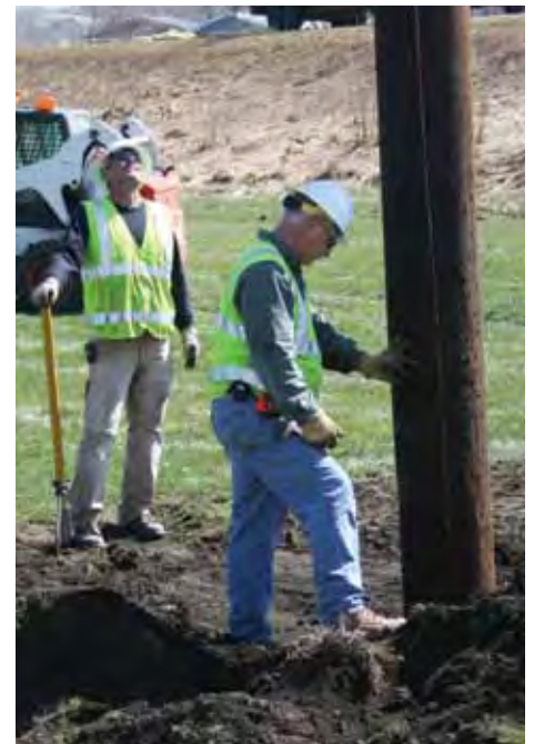
Linemen Gerry Freml, left, and Steve Harringa position the first of eight replacement poles at Mapleton.
