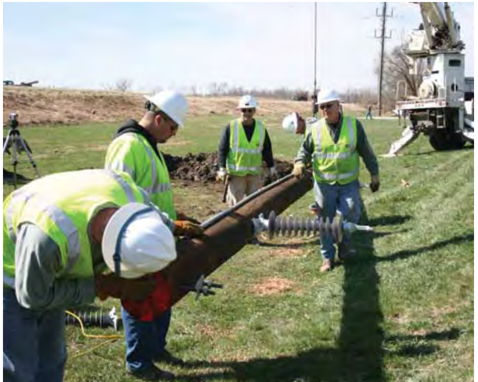
NIPCO engineering assistant Chad Barthman, left, and linemen Jim Marco, Gerry Freml, Terry Madsen and Steve Harringa, prepare a new pole to be set on the outskirts of Mapleton where a tornado tore out eight poles and broke conductor. NIPCO facilities sustained about $150,000 in damage.
